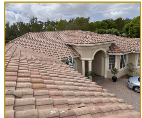
Hurricane Damage - Wellington
