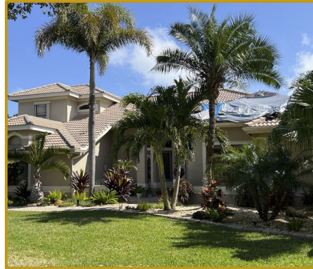
Hail and Wind Damage - Indialantic
