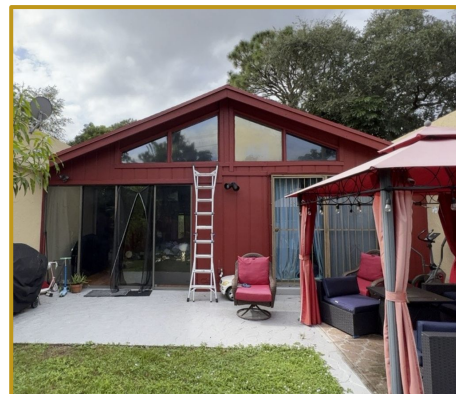
Wind Damage - Fort Lauderdale
